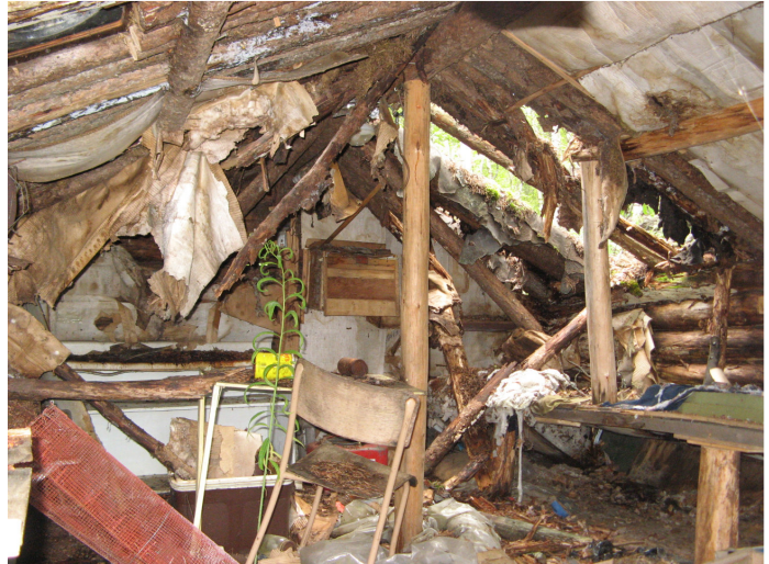
Inside trap cabin
